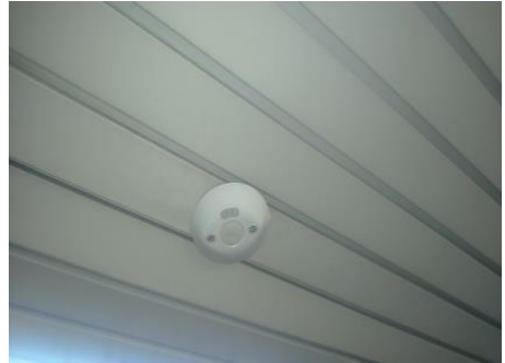
Provision of Occupancy sensors
