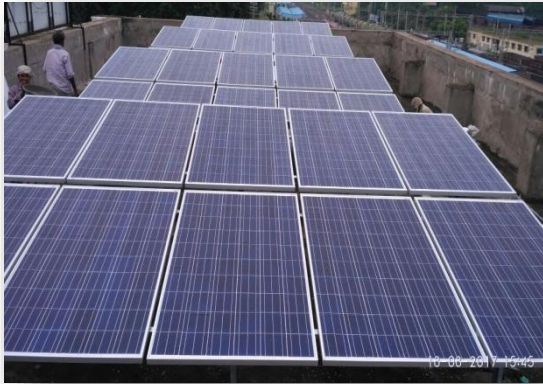
On site 90 kWp solar plant,
