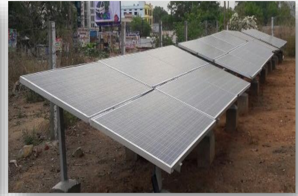
5 HP solar pump panels
