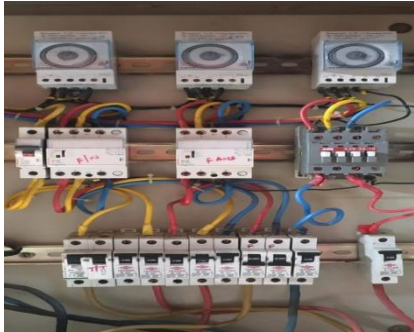
Provision of Timers for 30% & 70% fans and lighting circuits
