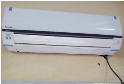
Energy efficient inverter type AC units
