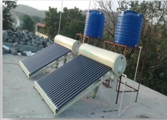
2000 LPD solar water heating system,
